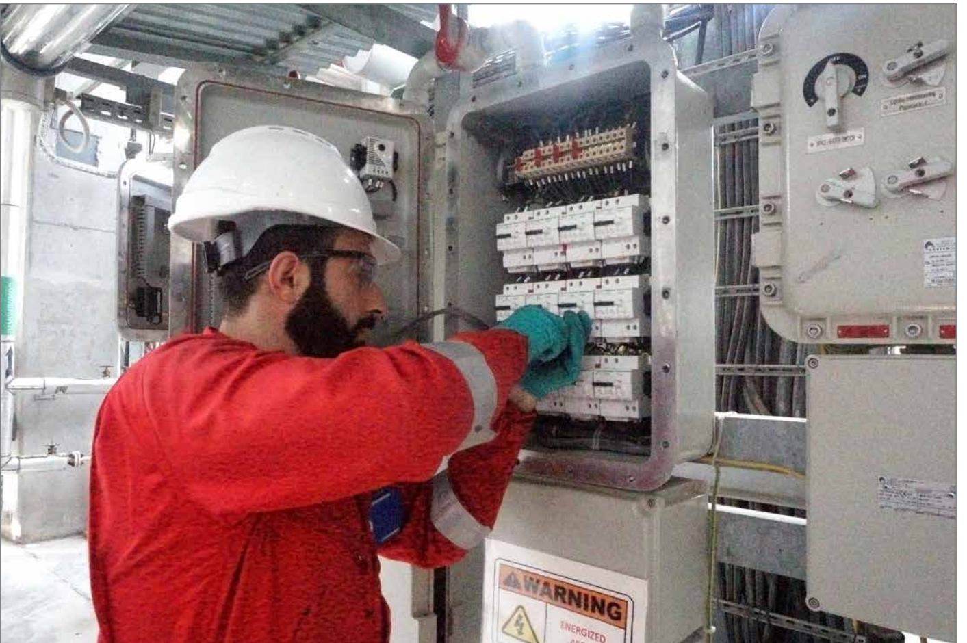
Maintenance of electrical distribution boards
