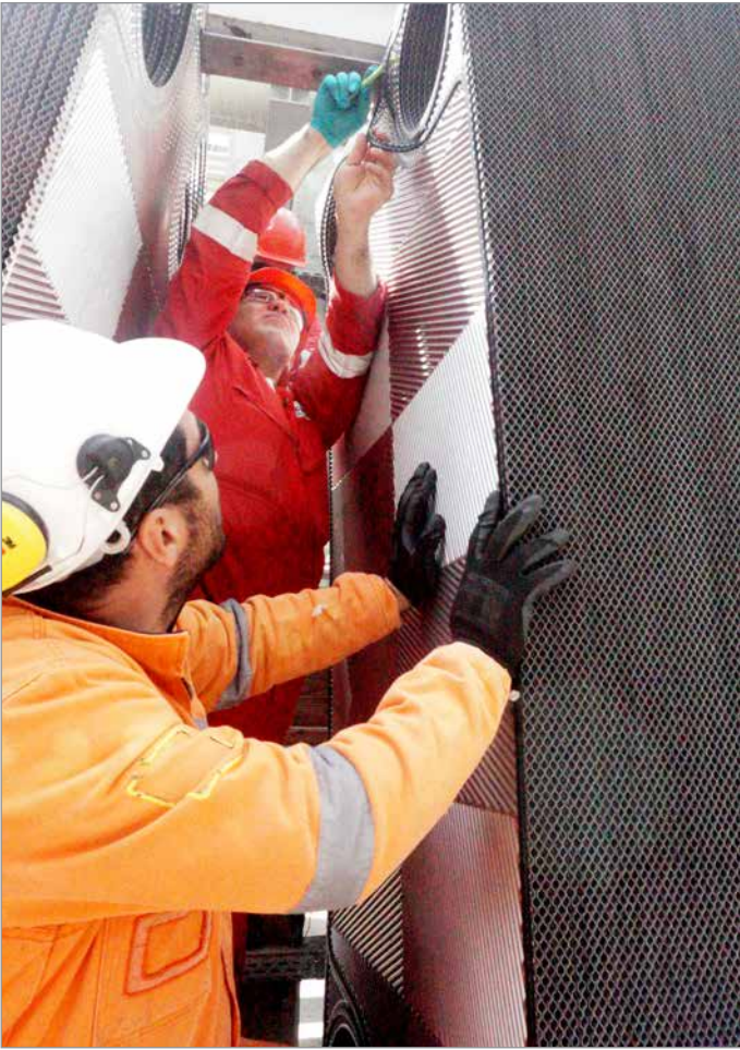
Heat exchanger plates reassembled into packs
