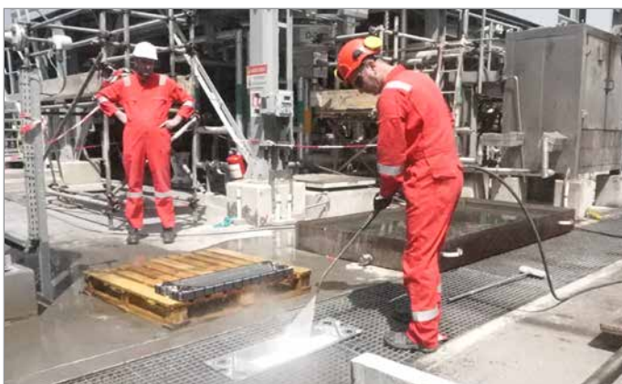
Rinsing of cleaned heat exchanger plates
