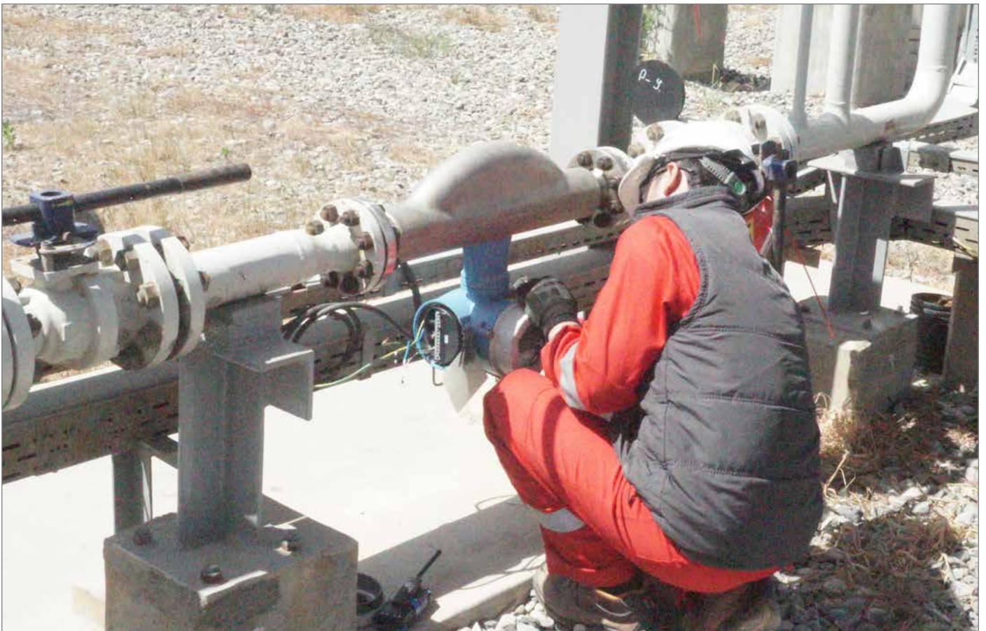
Inspection, maintenance (cleaning), and troubleshooting of Coriolis mass flowmeters to ensure measurement accuracy and long-term consistent operation
