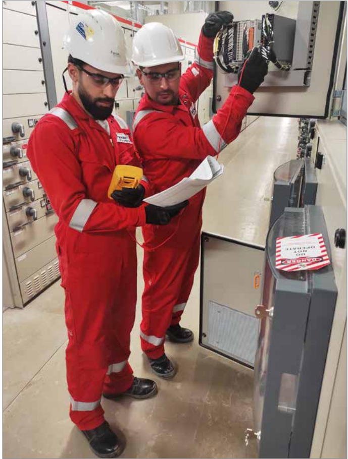
SAKHAVAT RAFIYEV ELECTRICAL SUPERVISOR ENGINEERING & MAINTENANCE DPMT
