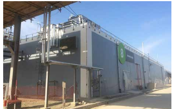
PP/U&O: Common Control Room. Punch List closing in progress
