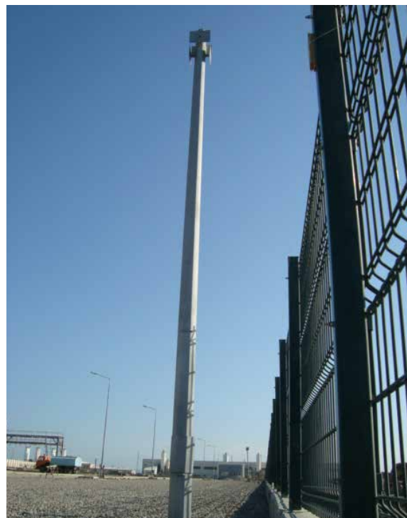
Permanent PS System. Casting of concrete foundations for camera poles. Cable pulling commenced
