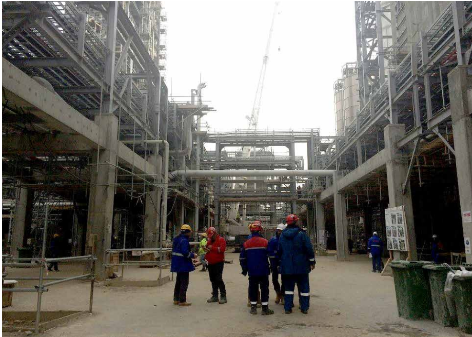
HDPE: Polymerization Pipe Rack.
