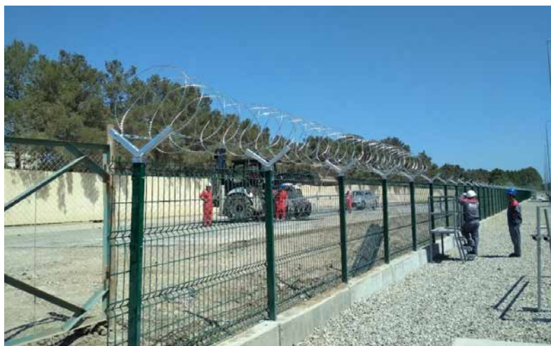
Razor Wire on the Perimeter Fence. Razor wire fabrication and installation in progress
