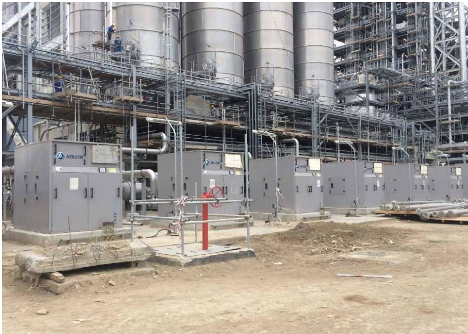
HDPE: Pellet blower package space for logistic conveying.
