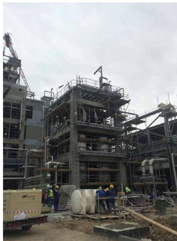
HDPE: Ethylene Treatment. Equipment Insulation completed on E-1423, D-1901 and E-1901 units
