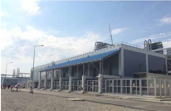
PP/U&O: Electrical substation. Punch List closing in progress
