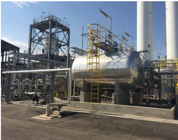
PP/U&O: Air/HP Nitrogen Condensate Compressor Station's Storage & Pumping facilities. Punch List closing in progress
