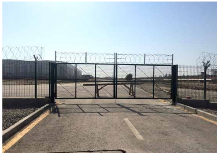
Razor Wire on the Perimeter Fence. Razor wire fabrication and installation in progress
