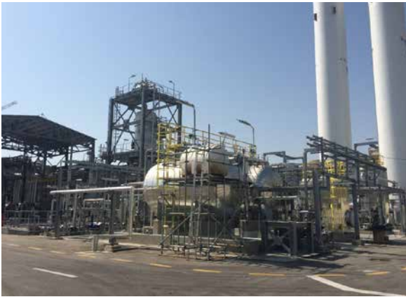
PP/U&O: Air/HP Nitrogen Condensate Compressor Station's Storage & Pumping facilities. Punch List closing in progress
