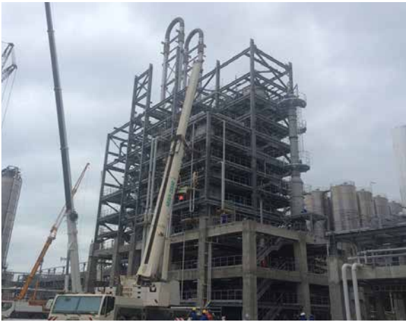
HDPE: Polymerization. Equipment erected. Piping & Support erection ongoing. SS, junction box, lighting etc. installation in progress
