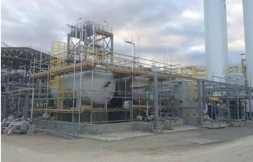
PP/U&O: Air/HP Nitrogen Condensate Compressor Station's Storage & Pumping facilities.
