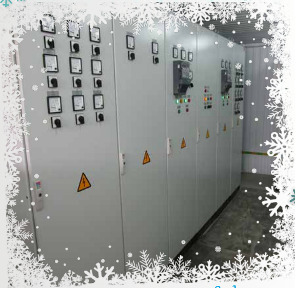
Energization of the Nitrogen Generation Unit
