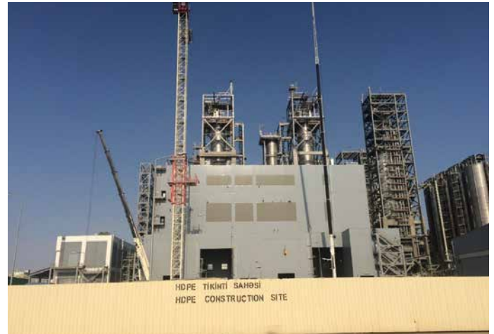
HDPE: Extrusion Building. Roof tiling completed. Sandwich panel installation mostly completed. Piping insulation ongoing. HVAC electrical cabling ongoing
