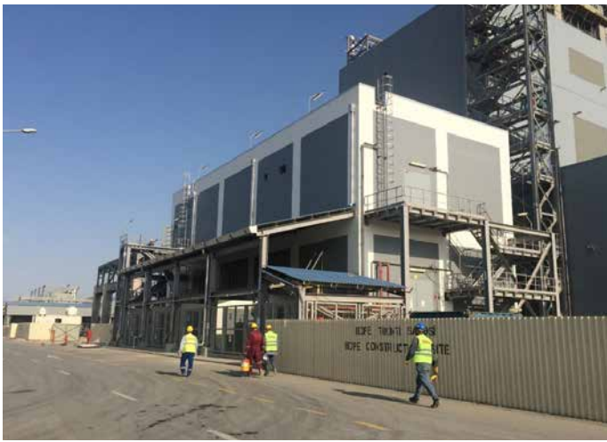
HDPE: Electrical Substation. Cabling and termination completed
