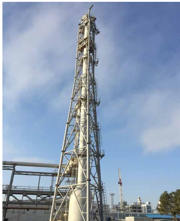
PP/U&O: Flare Stack. Piping and equipment testing started. Electrical and instrumentation works started
