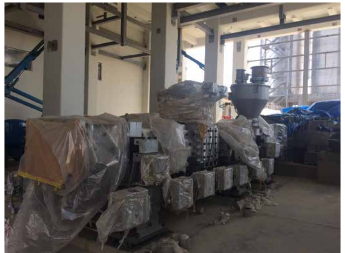
Extruder Package equipment. Extruder Package equipment (MARUBENI JSW, Japan) has been delivered to the site and is undergoing installation
