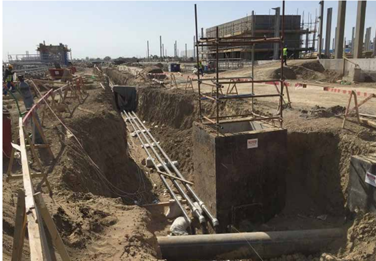
PP/U&O: UG installation. Pipe and manhole installation ongoing for RWS, SS, FW and POCS system
