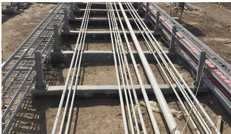
PP/U&O: Pipe Sleepers. Pipe erection and cable tray installation ongoing. Cable pulling started
