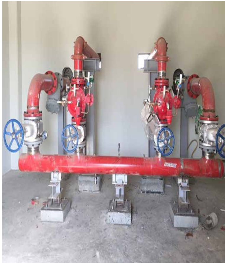
PP/U&O: Valve house.
