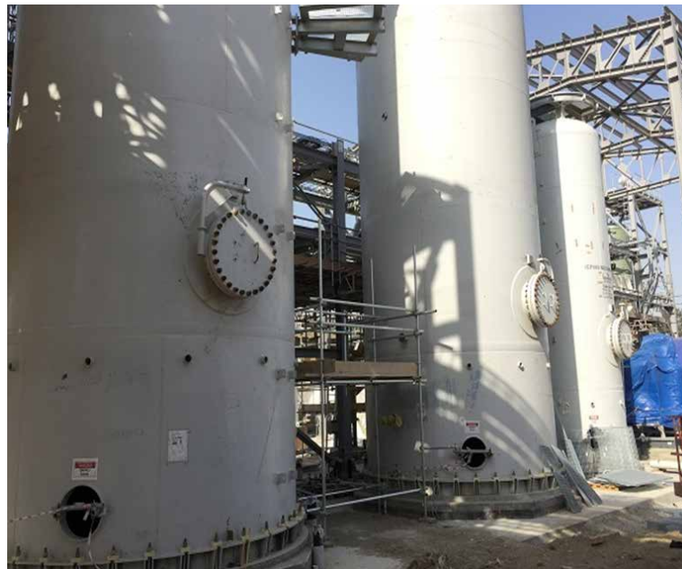
PP/U&O: Air/HP Nitrogen Condensate Compressor Station Storage & Pumping. Equipment and pipe alignment started
