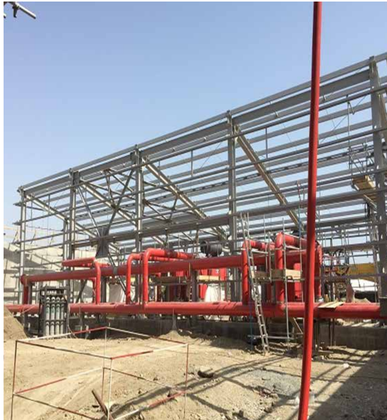
PP/U&O: Fire water Retention Basins and Pump House. Pump and pipe installation ongoing. Roof insulation started
