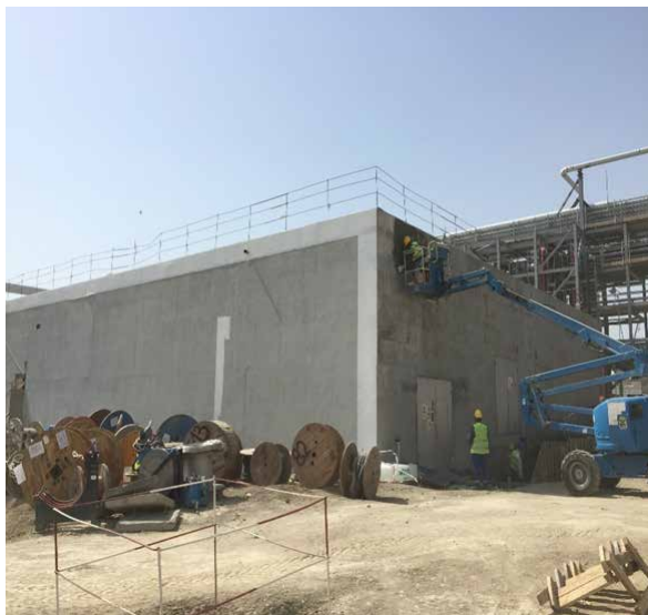
PP/U&O: Common Control Room. Panel and cable installation ongoing. Façade painting completed
