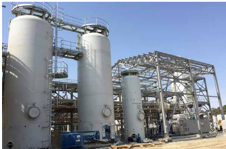
PP/U&O: Air/HP Nitrogen Condensate Compressor Station Storage & Pumping. Equipment and pipe alignment ongoing
