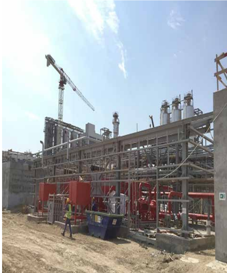
PP/U&O: Fire water Retention Basins and Pump House. Pump and pipe installation ongoing. Roof insulation ongoing
