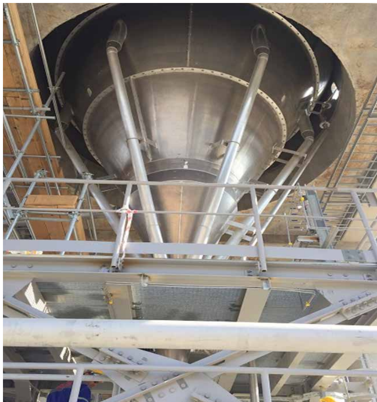
PP/U&O: Homogenization / Blender Silo. Pump, pipe and equipment alignment ongoing. Instrumentation installation started
