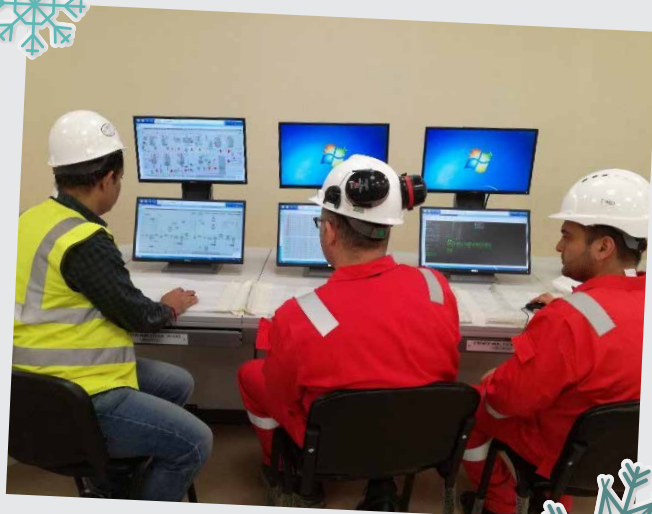
Control room screens go live
