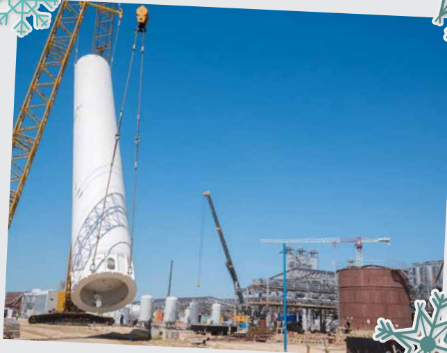
Liquid Nitrogen Storage and Gasification Unit
