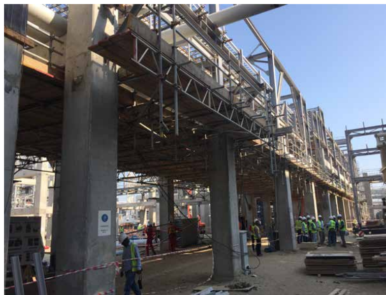
HDPE: Polymerization Pipe Rack. Pipe support installation ongoing. Cable tray installation started
