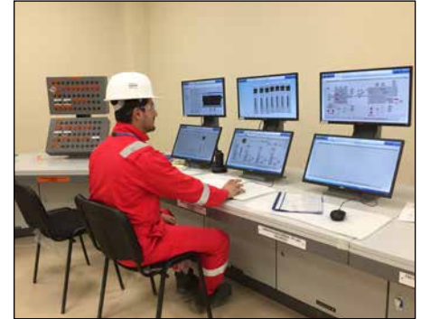
Control room screens now live p.19
